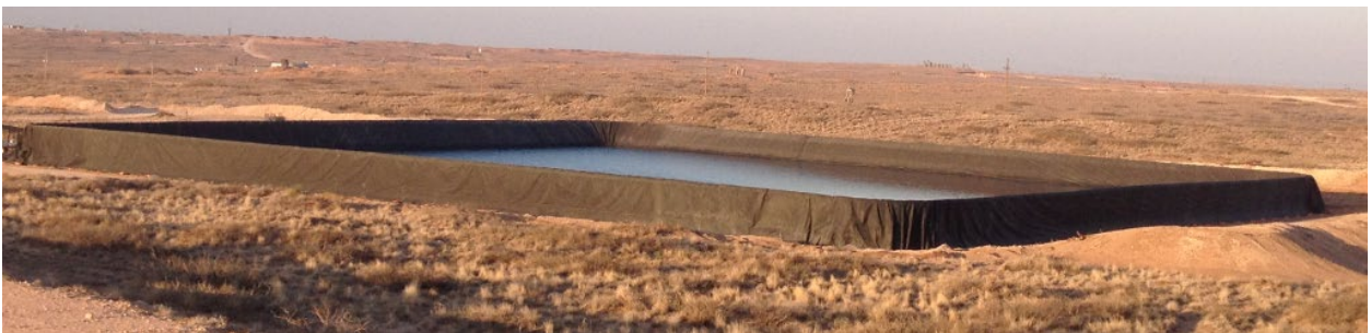
Figure 15: Photograph of a portable containment system (from Portadam).
