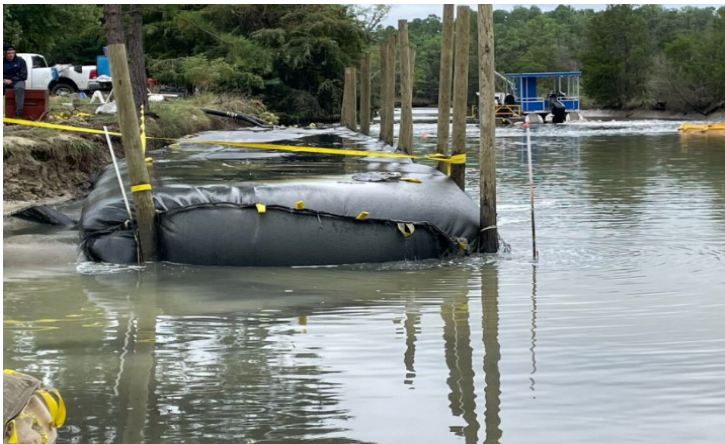
Figure 7 (above): Recently permitted and constructed project utilizing geotubes filled with dredged material in Gloucester. The tube has been covered with sand and grass and will function as a docking area at a public boat landing.
