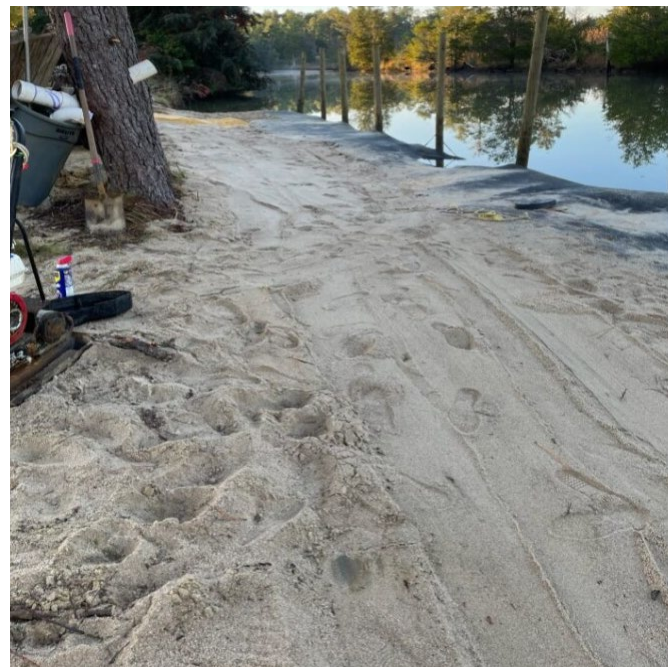
Figure 8: Recently permitted and constructed project utilizing geotubes filled with dredged material in Gloucester. The picture shows the tube as it is being covered with sediment. Grass has since been planted atop the tube and the site will function as a docking area at a public boat landing.
