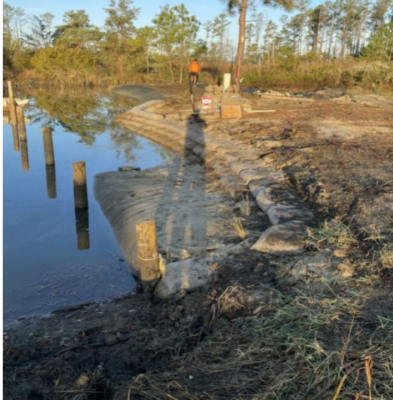
Figure 5 (above): Recently permitted and constructed project utilizing geotubes filled with dredged material in Gloucester. The tube has been covered with sediment and tidal marsh grasses have been planted atop the tube as part of a living shoreline.
